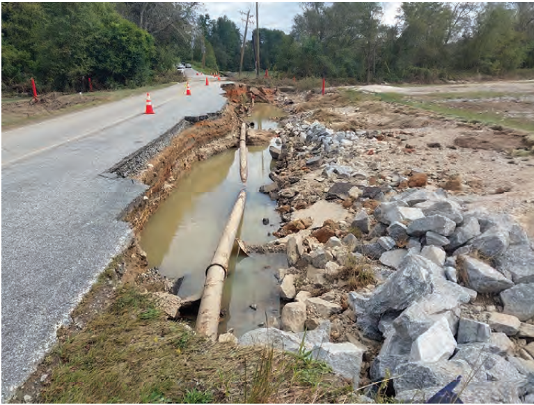
After Hurricane Helene in 2024, damage like this was common in the service area of the Hendersonville Water and Sewer Department. Most water customers had service restored in a few days.
