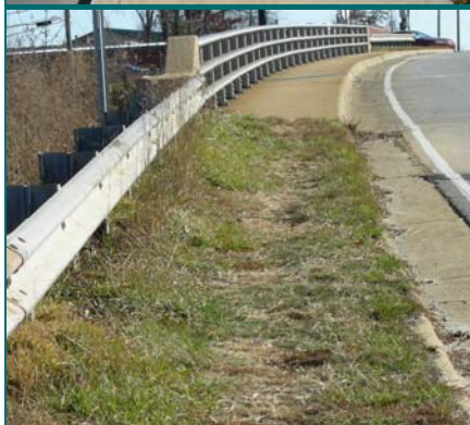
Sidewalk obstruction (top), lack of sidewalk continuity (bottom)
