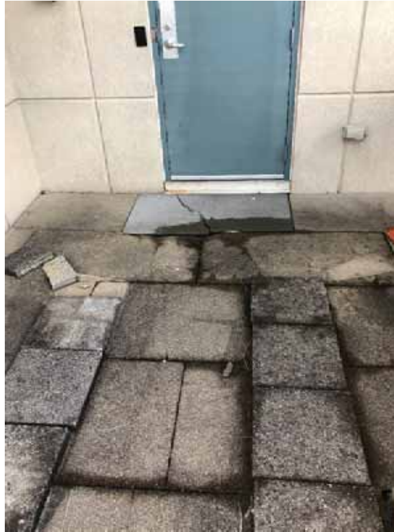
Photo 7 – Broken/missing insulation-paver blocks at porch
