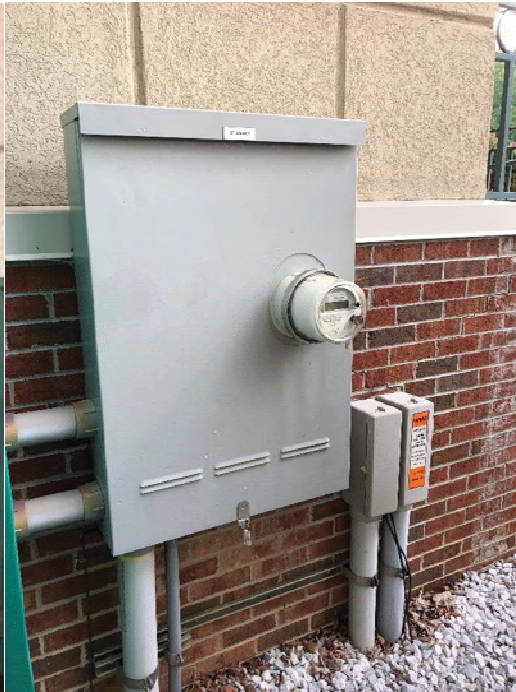
Meter Base and Fiber Entrance
