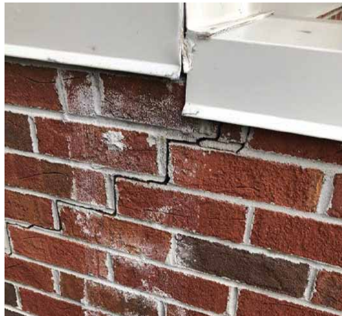
Photo 6 – Stepped crack in brick near generator
