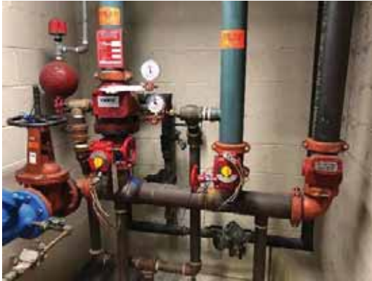
Sprinkler back flow (blue) and domestic back flow (below middle riser)
