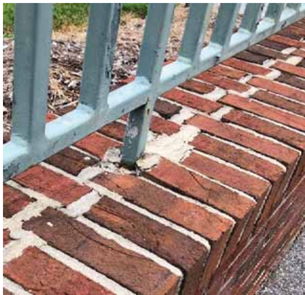
Photo 8 – Brick damage at rail connections
