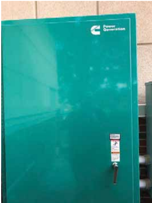
Outside Transfer Switch
