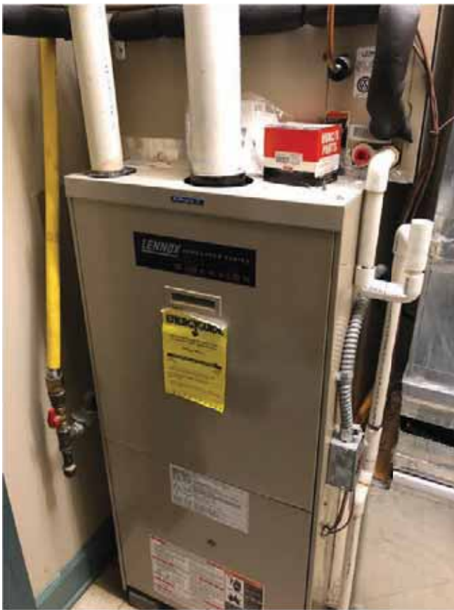
HVAC Indoor Units
