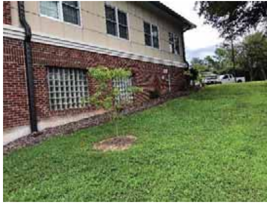
FDC upper end of building
