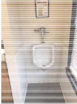
Flush valve urinal
