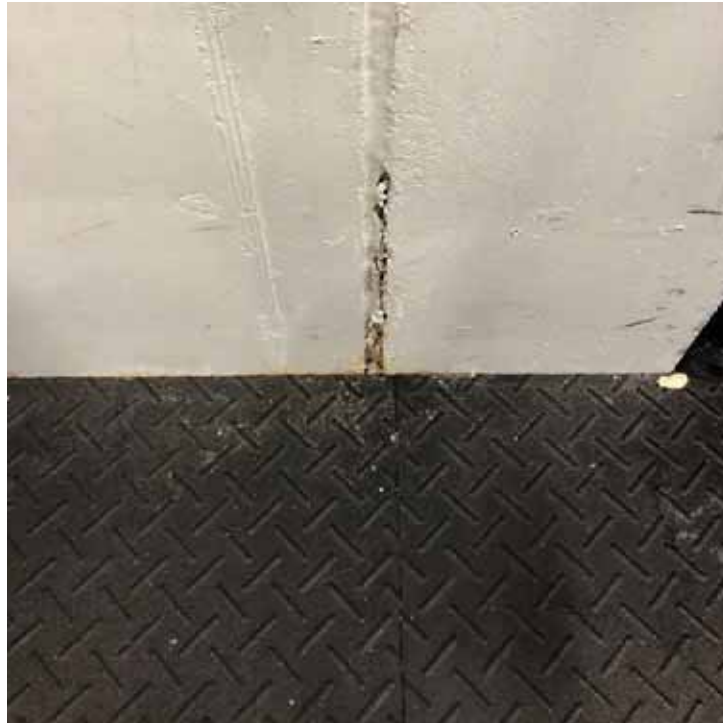
Photo 2 – Joint failure in fitness room
