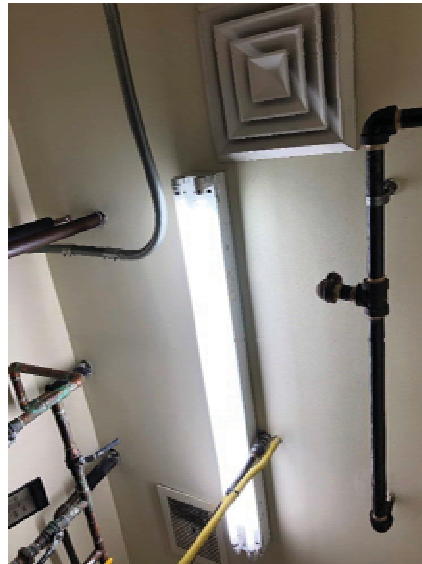
Few florescent lights remaining
