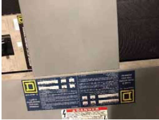
Square D I Line MDP Panel
