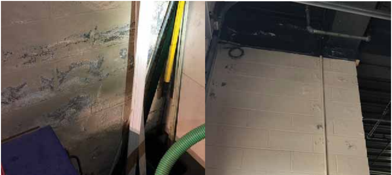
Photos 3 & 4 – Efflorescence on CMU walls in lower level
