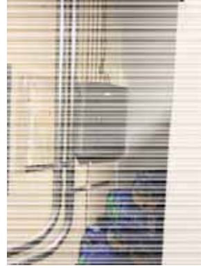
Original E Panel and old transfer switch location
